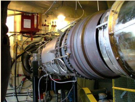
GM-Allison 501KB5 gas turbine first engine installed at N company in Kawasaki, 3MW Co-Gen Set
